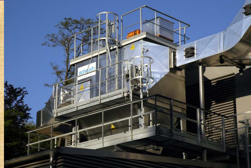
Electrostatic precipitator of a biomass heating system with a heat power of 2 MW
