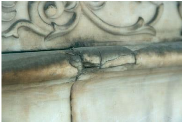
Figure 4.12.: Cracks caused by water run off. Credit?
